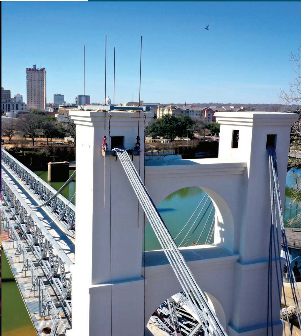
Rehabilitation on the historic Waco Suspension Bridge continued in 2021, with completion on schedule for 2022.
