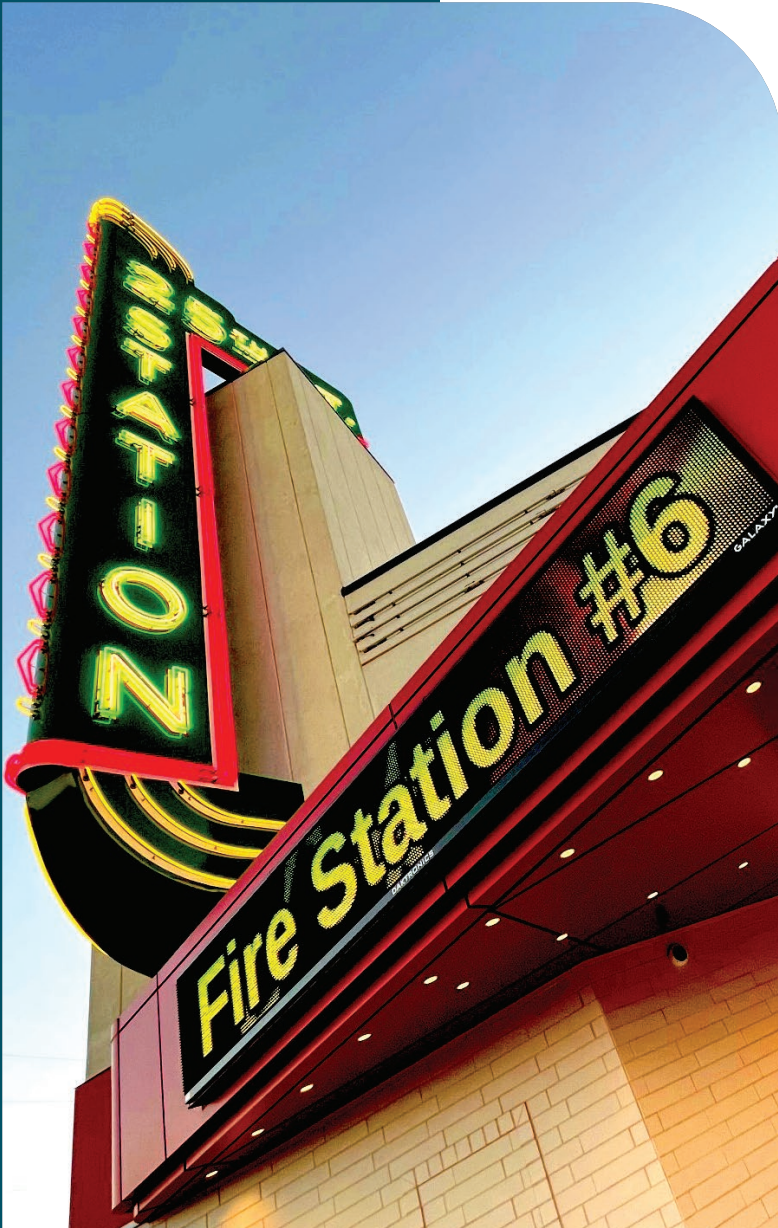
Fire Station #6 nears completion - November 2021. Located on the former 25th Street Theatre site, it will house fire administration and have a community room for the public to use.
