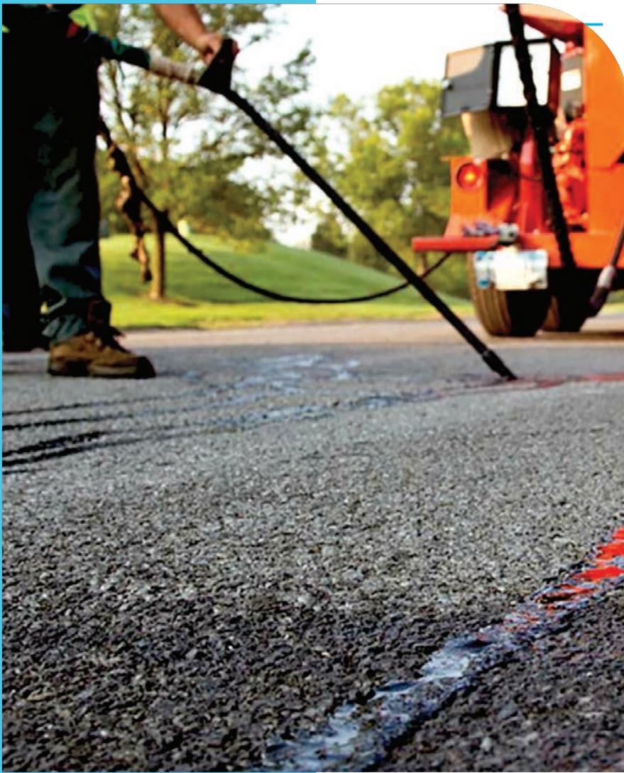
Crack sealing on multiple streets took place in 2021 and continues as part of the Better Streets Program.
