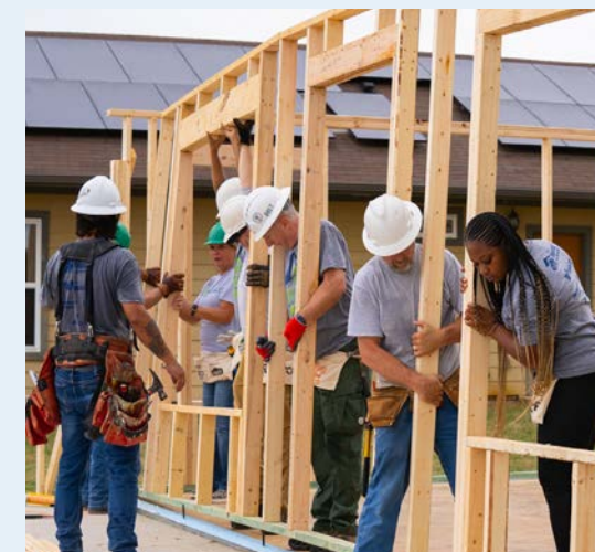
City of Waco staff volunteering at Habitat for Humanity's Raise the Roof program in October 2023.
