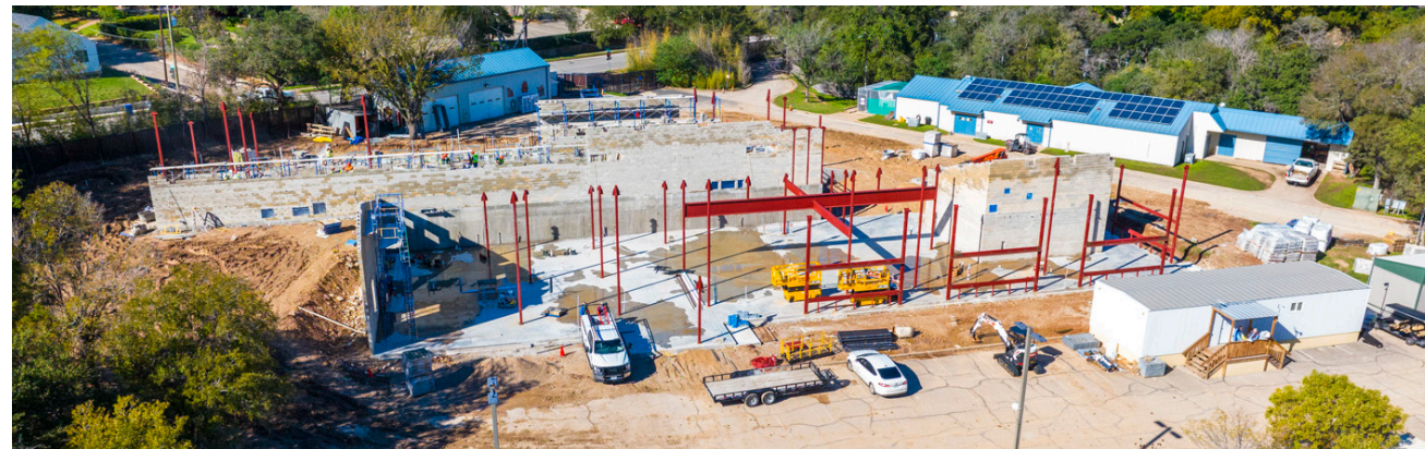
Penguin Shores exhibit, Education Center, and Veterinary Hospital Complex construction site in October 2023.
